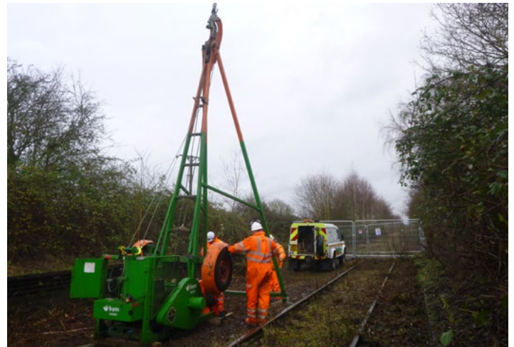
^ This cable percussive rig is being used to drill boreholes for geotechnical and water table surveys. Boreholes are typically 10 to 30 metres deep.
